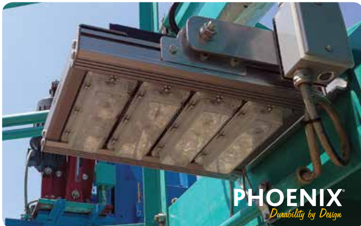
The cover photograph was taken at a port terminal in Malaysia. The EcoMod Series is shown on a Rubber Tire Gantry (RTG) crane.
