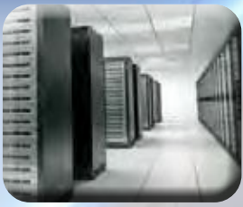
UPS & Data Centre
